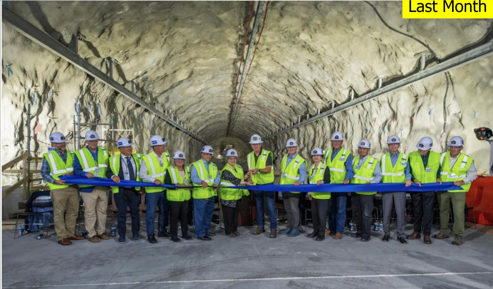
A ribbon-cutting event was held at the Sanford Underground Research Facility in Lead, S.D. to mark the completion of excavation work for LBNF/DUNE. Credit: Ryan Postel
